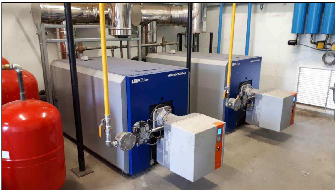
Figure 1 : Local 1 – chaudières gaz propane 300 kW (x2)
