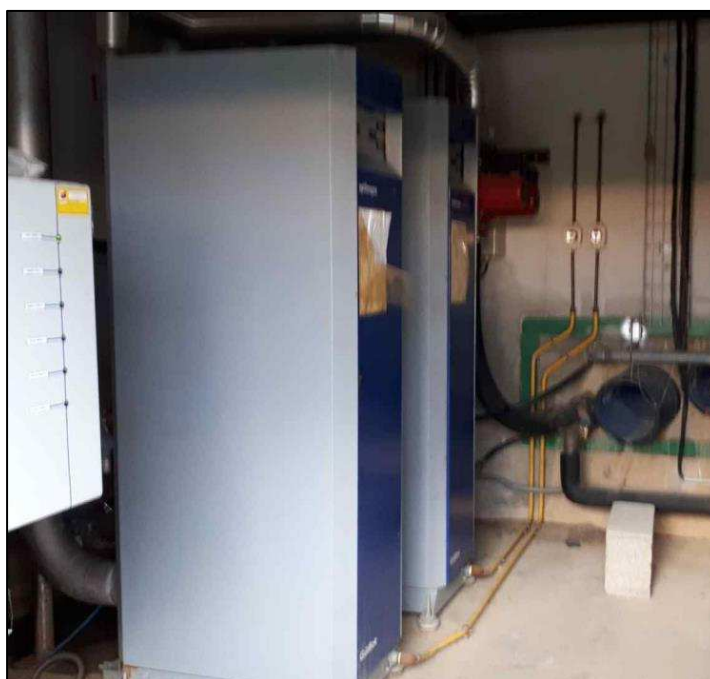
Figure 2 : Local 2 – chaudières gaz propane 90 kW (x2)
